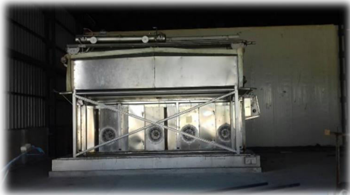
IQF Plant of 2MT/hr
