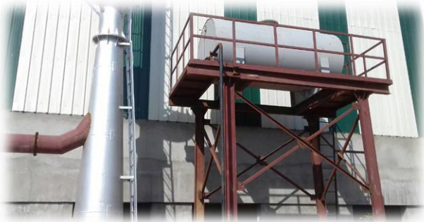
Boiler at Samba DC
