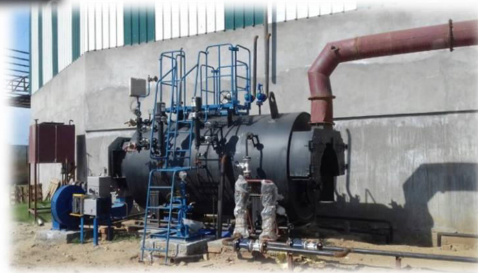
Boiler for blanching of vegetables
